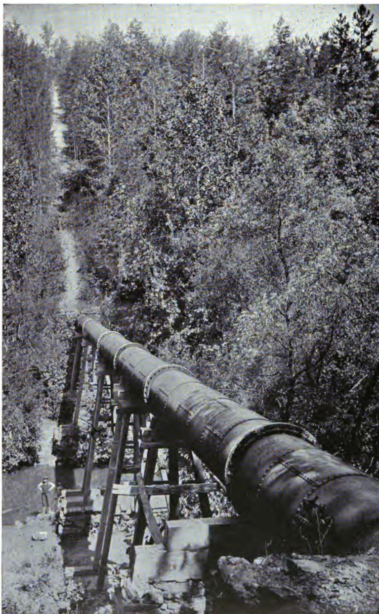
WROUGHT-IRON SIPHON PIPE (3 FEET INSIDE DIAMETER), 2000 FEET LONG, ON THE HAND BARLOW DITCH LINE, CROSSING THE YAHOO LAH RIVER. ONE MILE FROM DAHLONEGA, GA.
